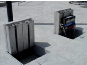
Piazza 700 – Waste water shaft and energy supply system
