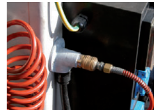
Compressed air connection
