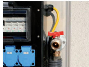
Fresh water connection with freeze protection by heating band
