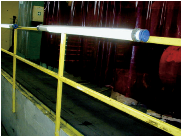
Handrail illumination, Austrian Railways
